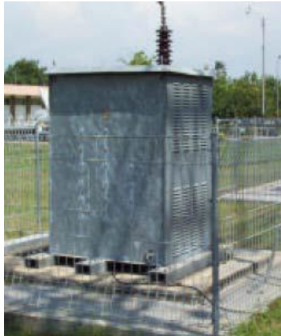
Gambar 2. 10 Neutral grounding resistance (NGR)
