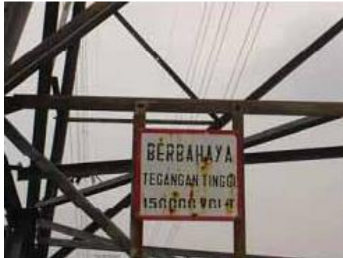
Gambar 2.15. Rambu Tanda Bahaya Tower
