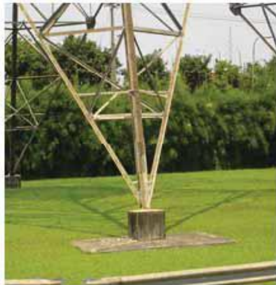
Gambar 2.12. Pondasi tower ( lattice ) SUTT 500 kV
