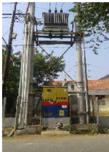
Gambar 2.10 Gardu Distribusi Tipe Portal
