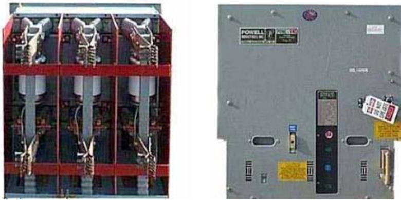
Gambar 2.14 VCB (Vacuum Circuit Breaker)
