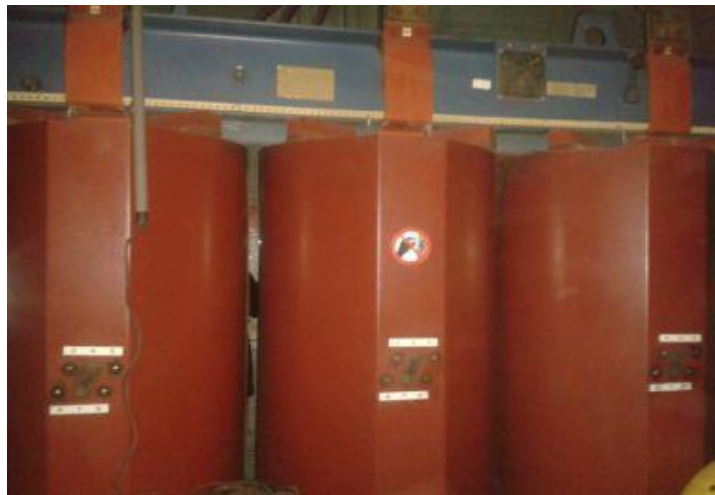
Gambar 2.21 Unit Auxilliary Transformer (UAT)
