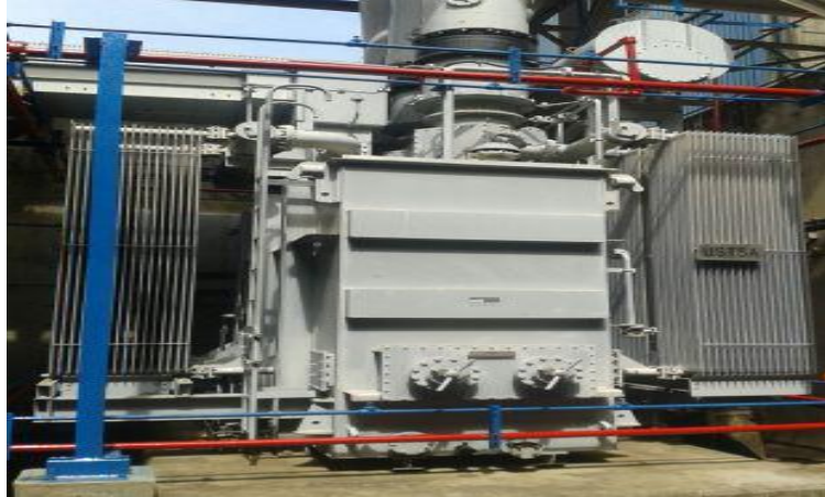
Gambar 2.19 Unit Station Transformer
