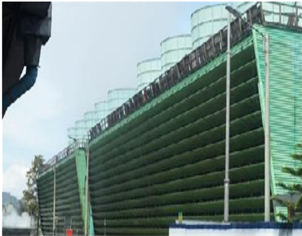
Gambar 2.11 Cooling Tower PLTP Kamojang
