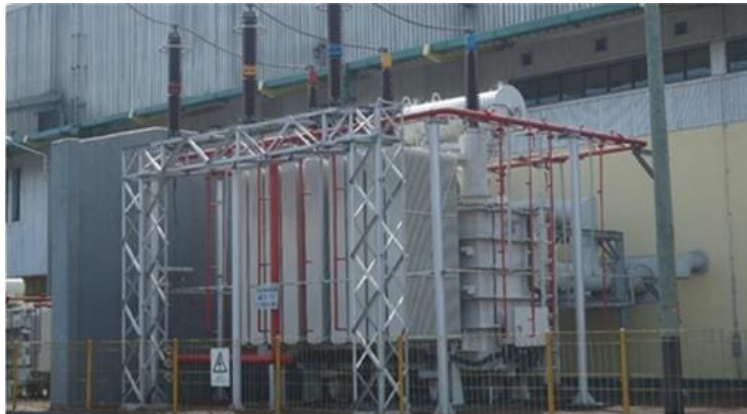
Gambar 2.13 Main Transformator 11,8 kV /150 kV
