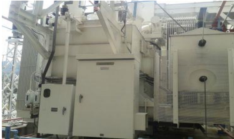
Gambar 2.20 Station Service Transformer
