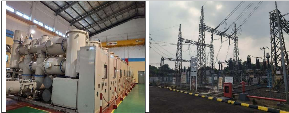
Gambar 2.1 Mixed Technology Switchgear di GIS Durentiga (Sumber: Dokumen Pribadi)
