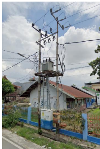
(a) Gardu distribusi portal
