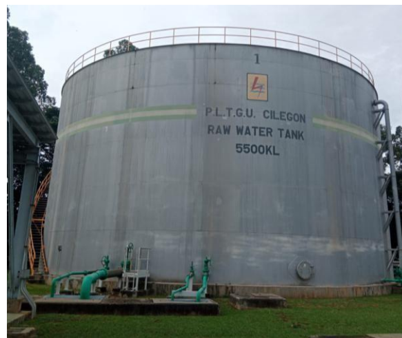
Gambar 2. 5 Raw Water Tank
