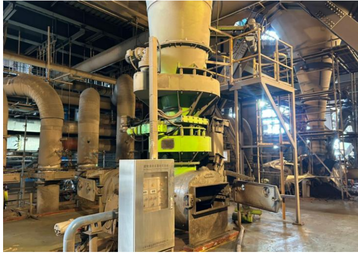
Gambar 2.12 Rotary Antiblocking System PLTU Labuan
