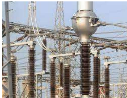
Gambar 2. 7 Current Transformer (CT)
