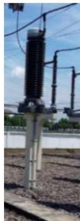
Gambar 2. 5 Potensial Transformator (PT)
