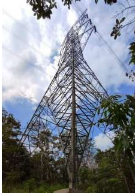
Gambar 2. 3 Tower Transmisi 150 kV
