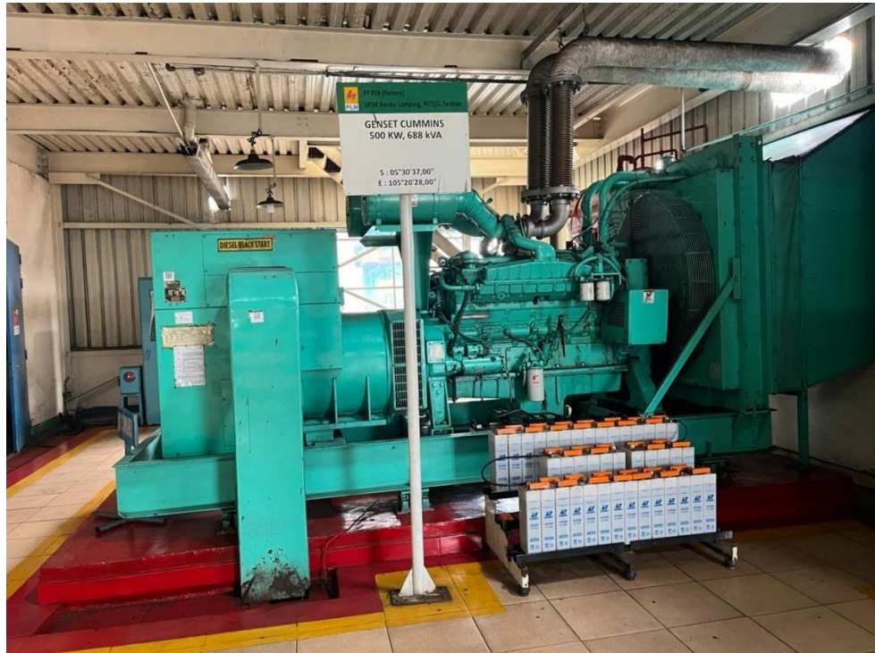
Gambar 2.2 Emergency Diesel Generator PLTD/G Tarahan
