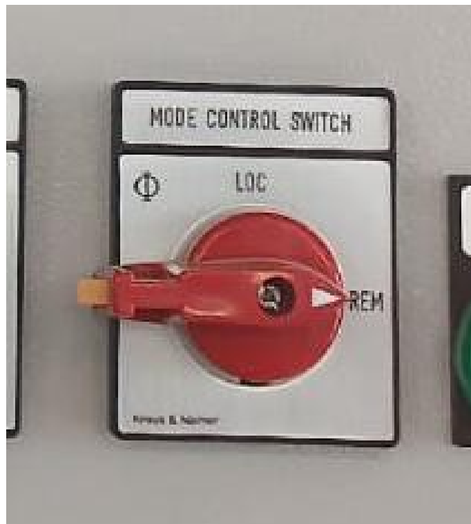
Gambar 2. 6 Selector Switch Remote/Local
