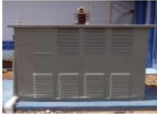
Gambar 2. 5 Neutral Grounding Resistance
