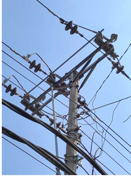
Gambar 4.16 Air Break Switch (ABSW)
