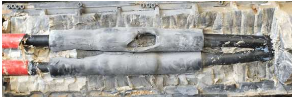
Gambar 2. 10 Dampak Partial Discharge
