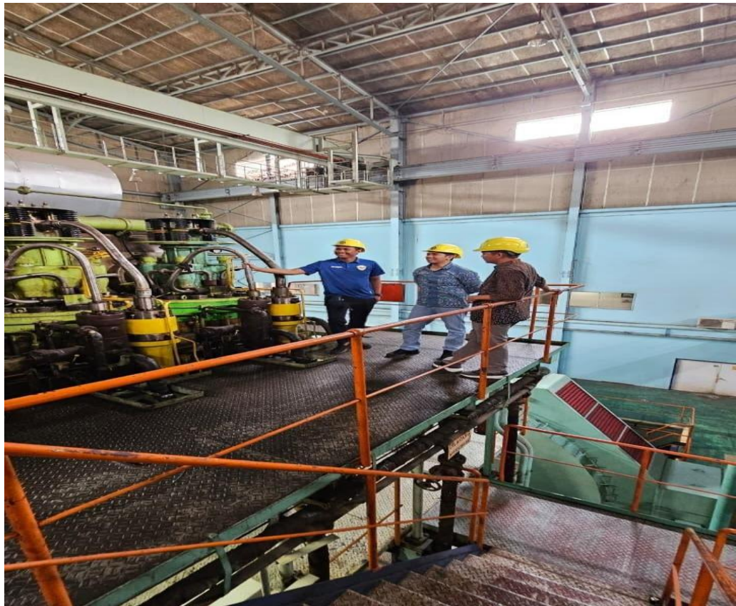
Gambar 2.3.1 Mesin Diesel ( Prime Mover )
