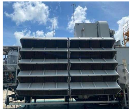
Gambar 2.11 Air Intake Pre-Filter
