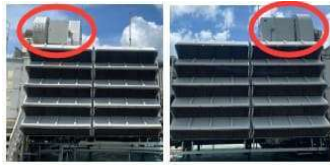
Gambar 2.10 Motor Ventilation Air
