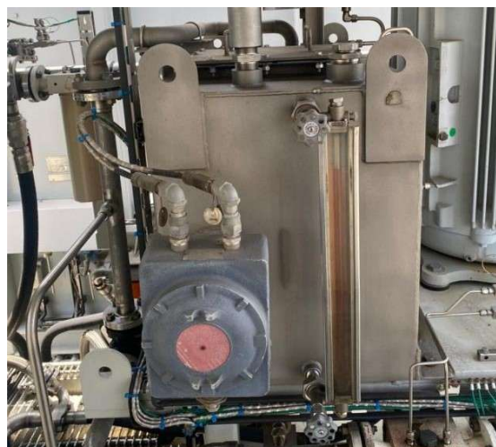
Gambar 2.8 TLO ( Turbine Lube Oil ) Reservoir PLTG MPP
