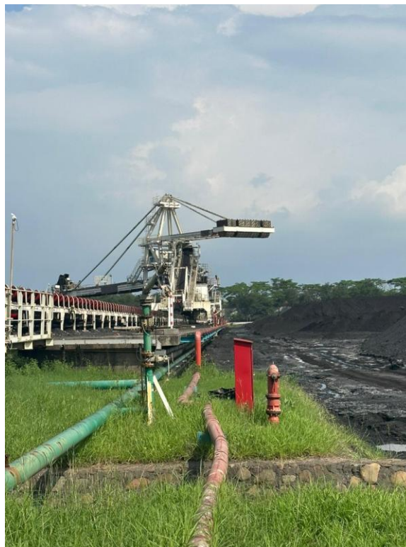
Gambar 1.2 Instalasi Pipa Penanganan Debu Batubara di Coal yard
