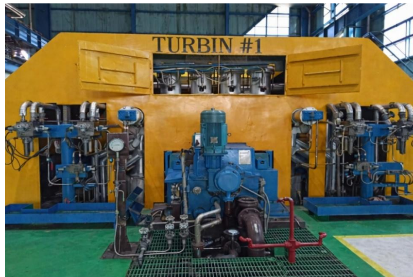
Gambar 7 Turbin Uap PLTU Ombilin Unit 1
