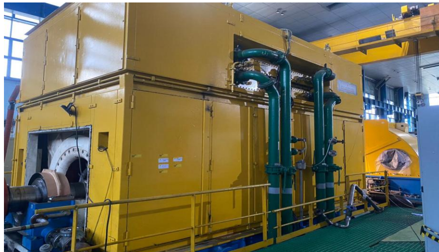
Gambar 8. Generator PLTU Ombilin Unit 1
