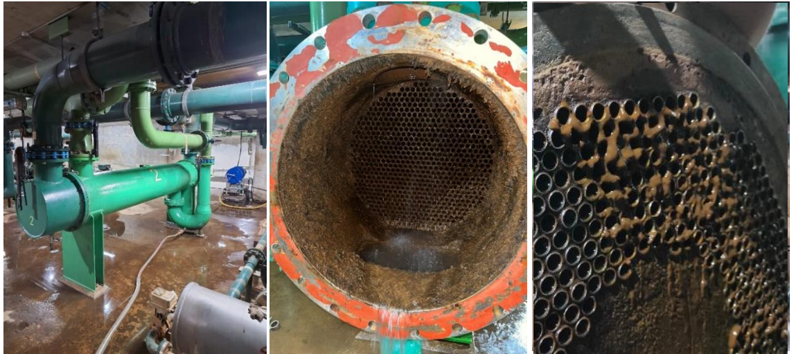
Gambar 1.3 Water Heat Exchanger PLTA Kotopanjang
