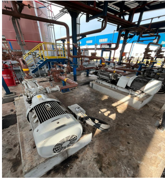
Gambar 2.17 Fuel Oil Supply Pump (Sumber: Dokumen Pribadi )
