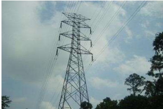
Gambar 2.7 Tiang penyangga (suspension tower) SUTT 150 kV
