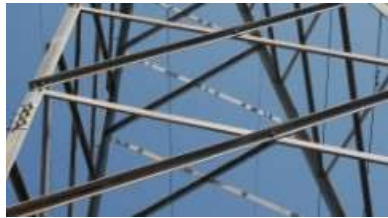
Gambar 2.3 Diagonal Tower Transmisi
