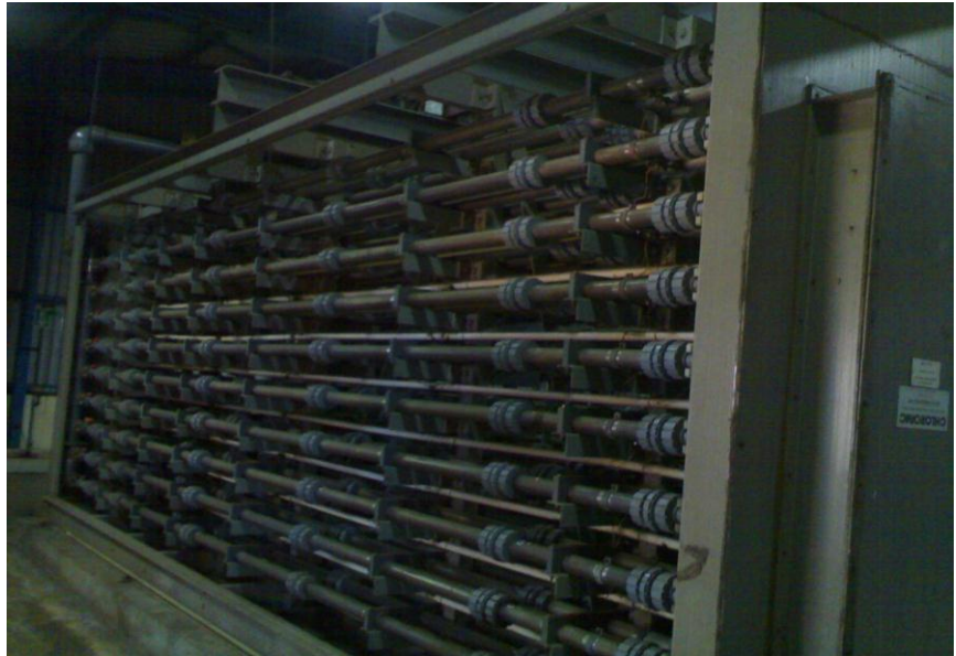
Gambar 2.8 Chlorination Plant UPB Suralaya
