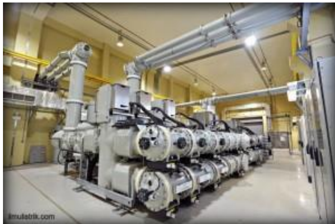
Gambar 2.4 Gardu Induk GIS (Gas Insulated Switchgear)
