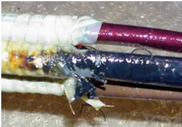
Gambar 2.4 Joint insulation contamination
