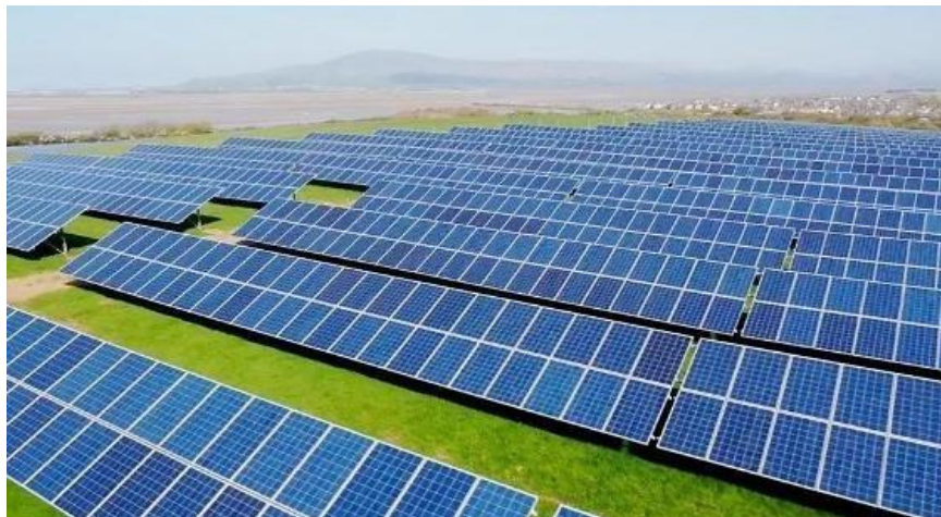
Gambar 2. 11 Ground Mounted Solar PV
