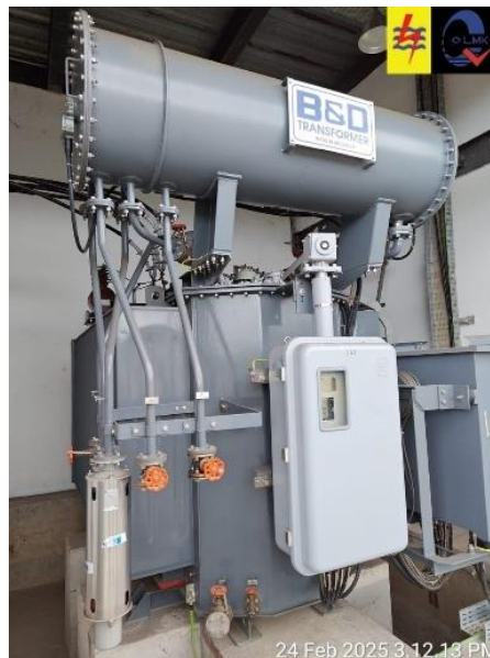
Gambar 2.1 Transformator GT PLTU Sofifi
