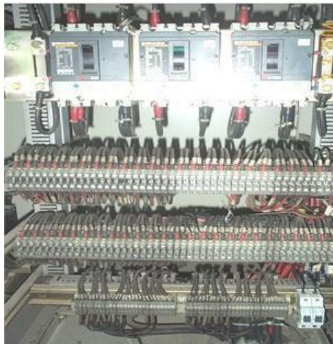
Gambar 2.2 DC Distribution Board
