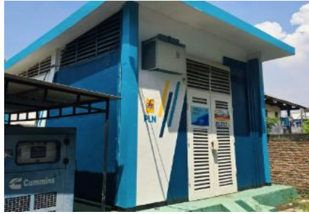
Gambar 2. 5 Gardu Distribusi Beton
