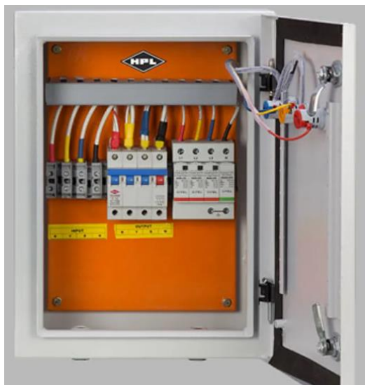
Gambar 2.6 AC Distribution Box
