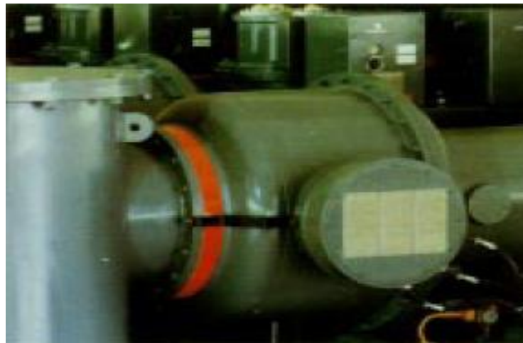
Gambar 2.3: Kompartemen Trafo Arus (model busbar 1 enclosure – 1 phase)
