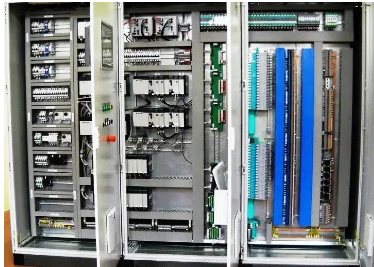
Gambar 2. 17 Distributed Control System (DCS)
