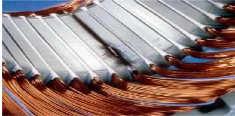
Gambar 2. 13 Broken Stator Winding
